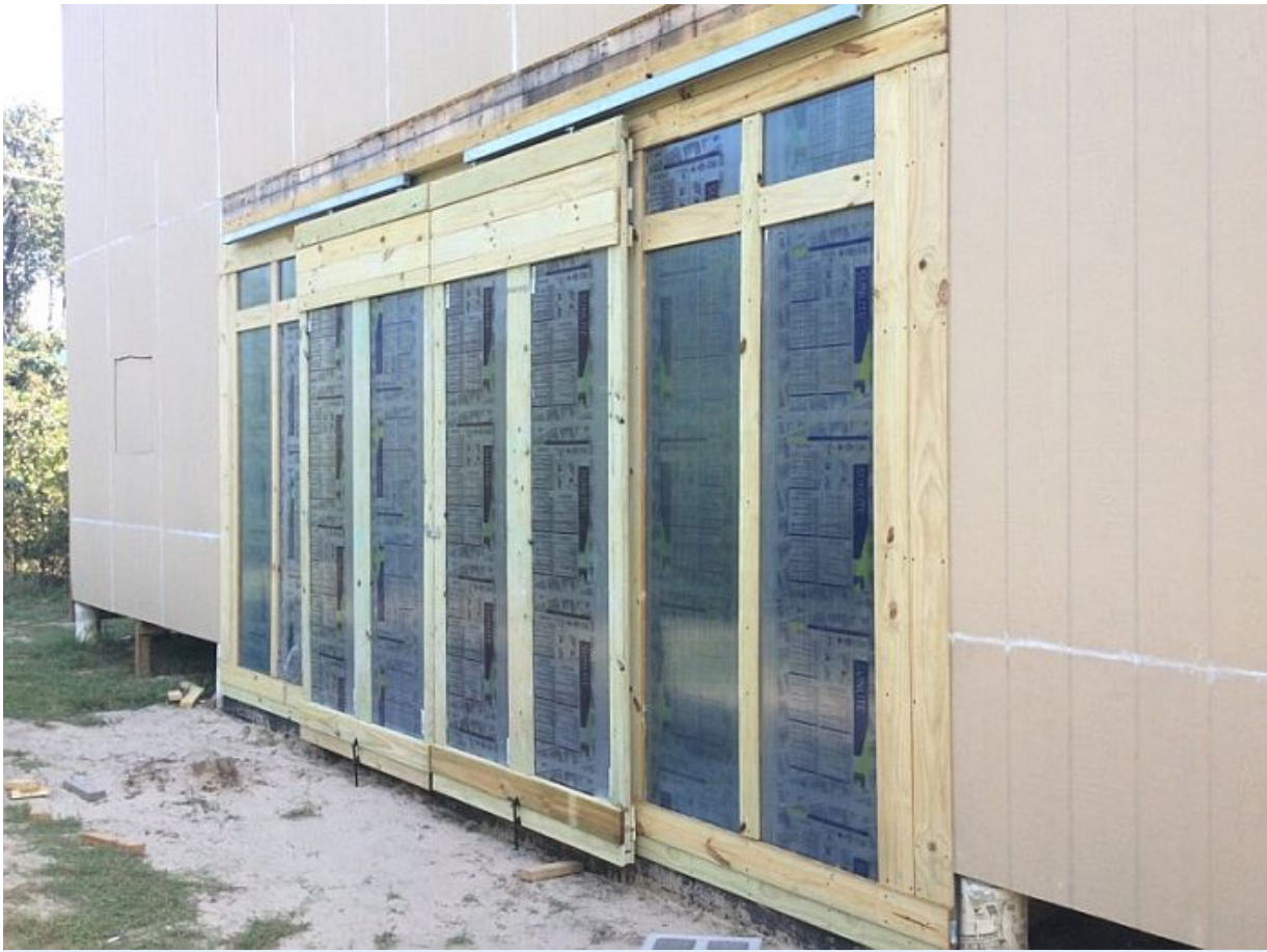
We just finished installing these sliding doors on the back of the shop!
